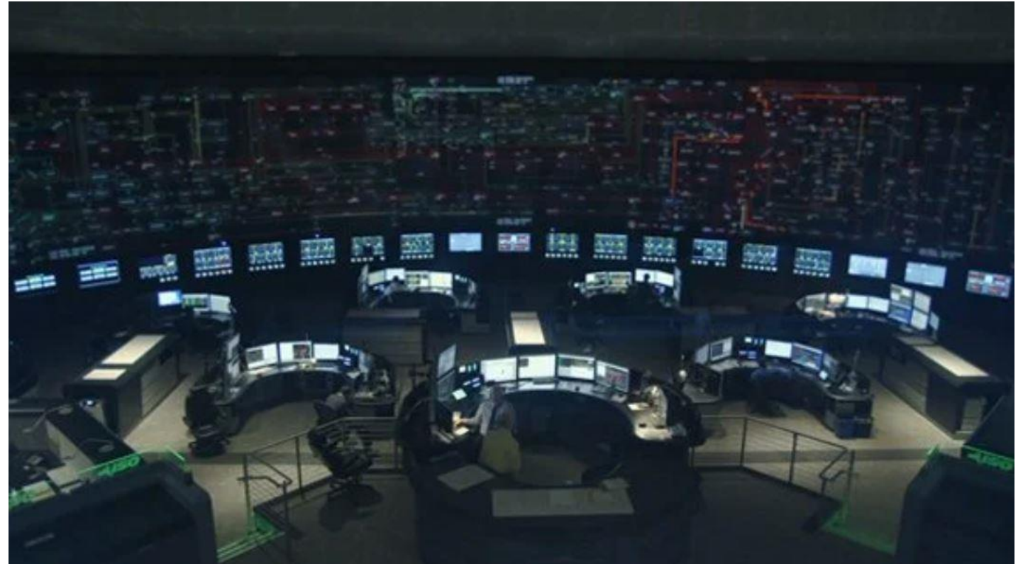
New York Independent System Operator (NYISO) control center
